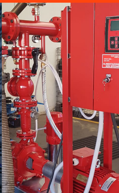
Fire protection systems
